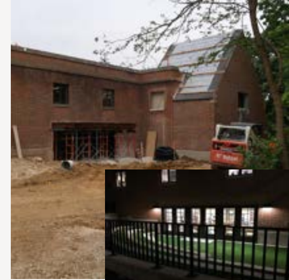
The Children's Terrace highlights the library's connection to neighboring Katharine Wright Park, bringing views of the park inside the library and creating a new library space for outdoor play and programs.
